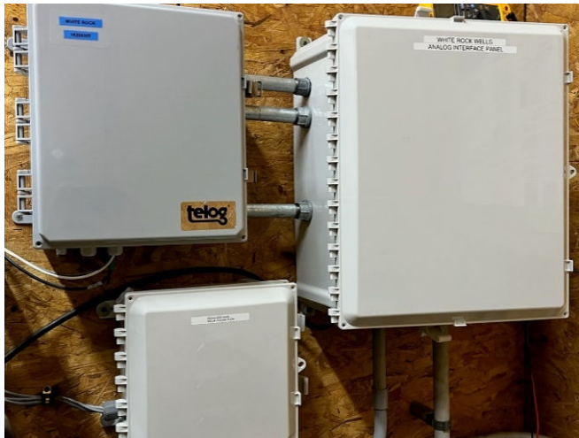
Electrical and telemetry panels
